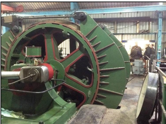
Forum members at their recent meeting at Papplewick Pumping Station, Nottingham
