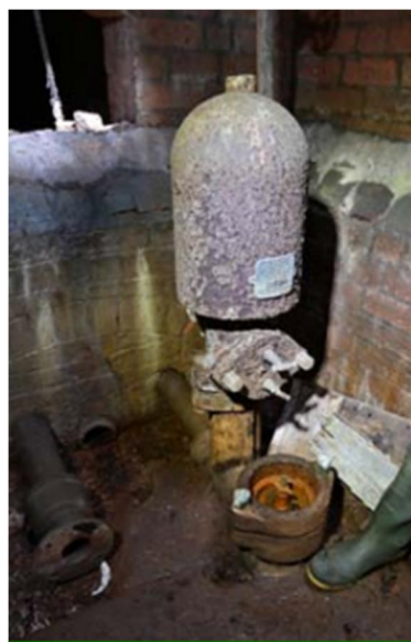
The surviving ram pump.
