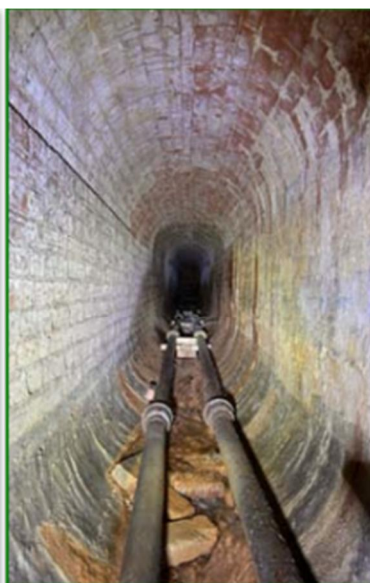
Feed pipes for the ram pump.
